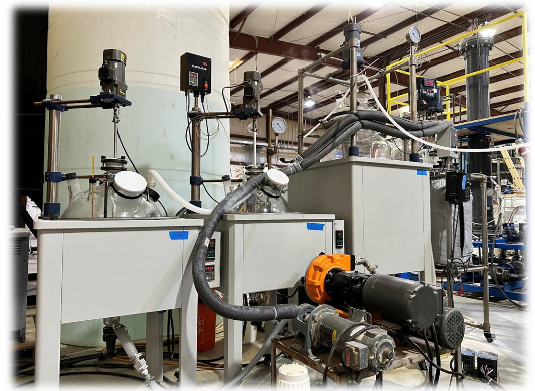
\text{Li}_2\text{CO}_3 circuit at Demonstration Plant
